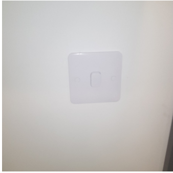
Electrical Switches Sockets/Power Points
