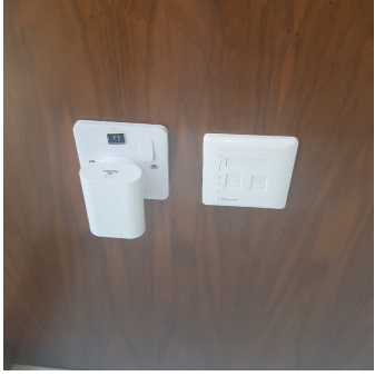
Electrical Switches and Power Points
