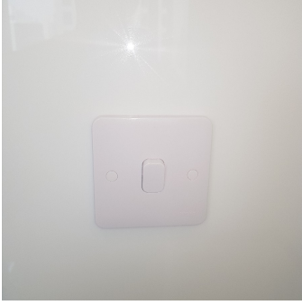
Electrical Switches and Power Points
