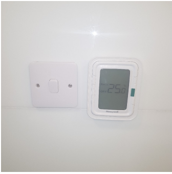
Electrical Switches and Sockets
